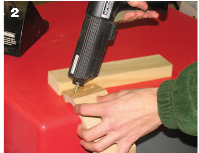
2 HiPURformer gun being used to attach a short molding - note the heat cradle at the upper left.
